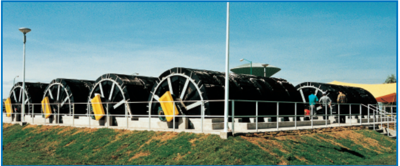
KEE Process Multiple 3.66m Diameter System in Mexico.
