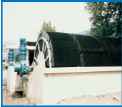
KEE Process Large RBC Modular System in France.
